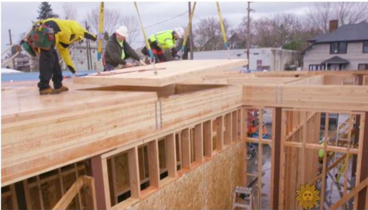
CLT panels are put into place at a construction site. / CBS NEWS
